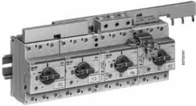
MS325 with auxiliary switch HK cross-wired with phase buses and power infeed block
