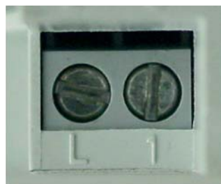
Figure 4. Modbus port terminals
